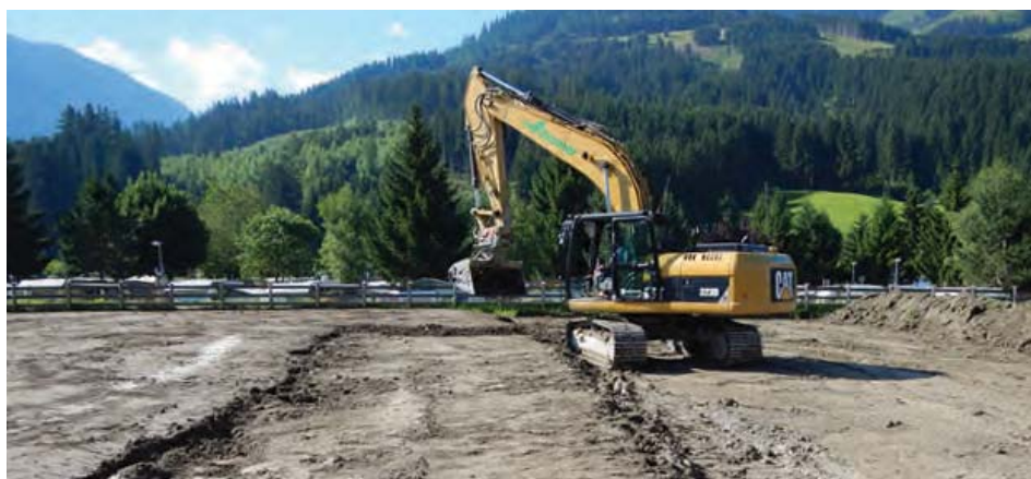
Figure 29: A positive example of soil treatment: The loosening of compacted soil followed by filling of underground and top soil in layers (Photo: Thomas Peham).
