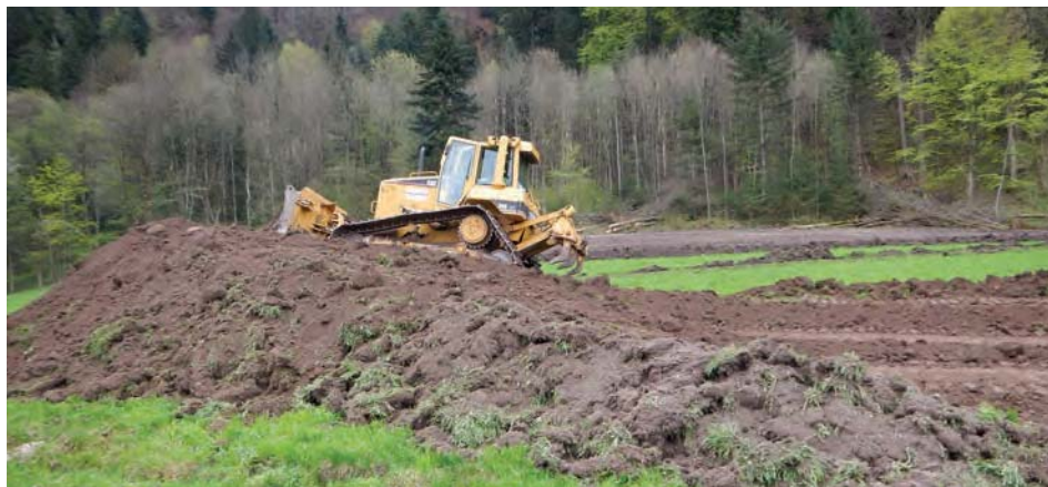
Figure 28: A negative example for soil excavation: No separation of turf, the high thickness of topsoil deposit and driving on deposit with heavy machinery (Photo: Thomas Peham).
